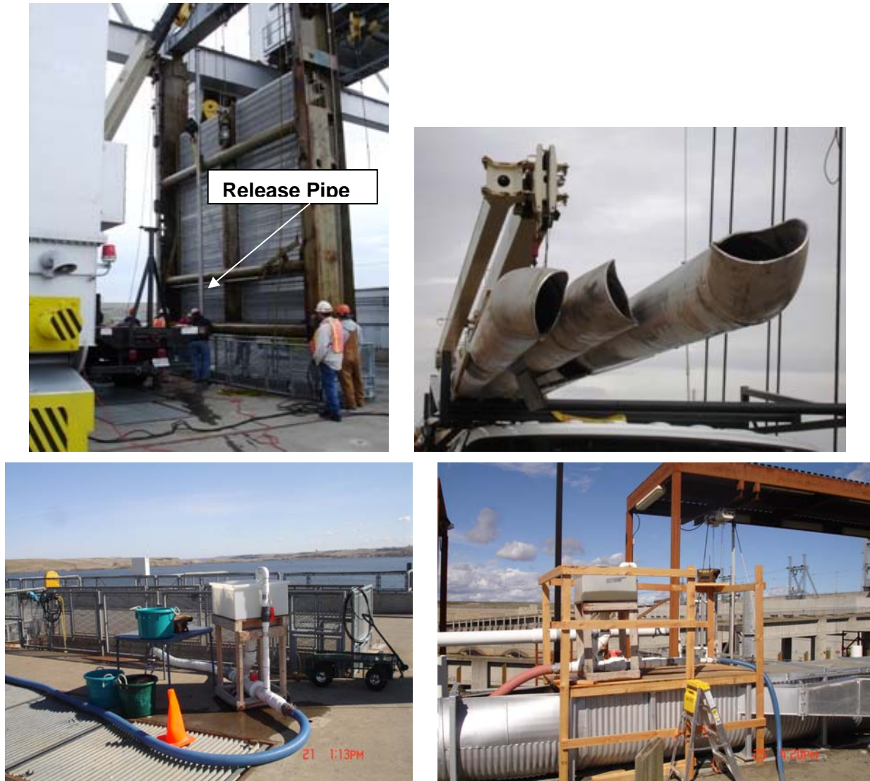
Figure 2-2 Release pipe attached to traveling fish screen frame (top left photo) 30-inch off-center toward North. Release pipes extended 3.2 ft below the screen frame in Slots A and B and 5 ft below frame in Slot C. Exit end of release pipes curved (top right photo) and oriented in a downstream direction when installed. Induction system (bottom left photo) carried test fish via a flexible hose to the release pipe. Induction system for control fish (bottom right photo) released fish directly into the exit flume of the Juvenile Fish Bypass Facility, Ice Harbor Dam, March 2007.
